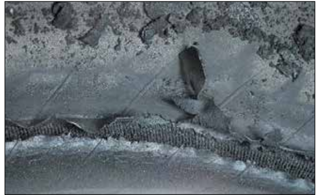
Inner Liner Damages
