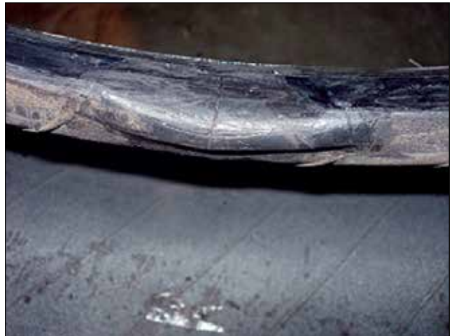
Bad Bead Repair
