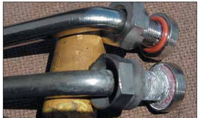
Note Corrosion On Bottom Valve
