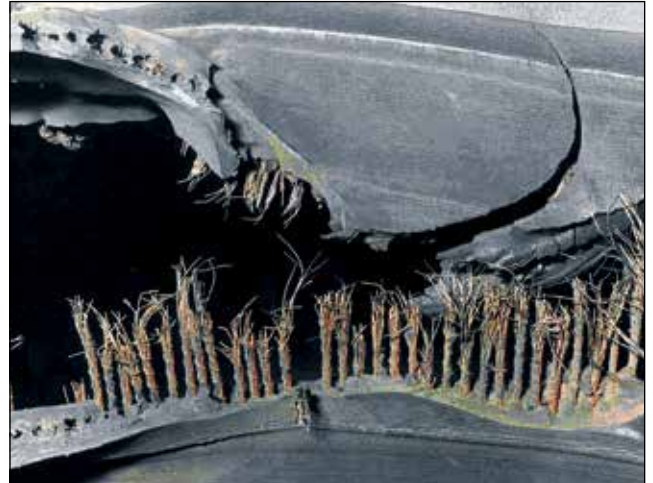
EFFECT: Any Damage That Will Allow the Casing to Oxidize CAUSE: Moisture
