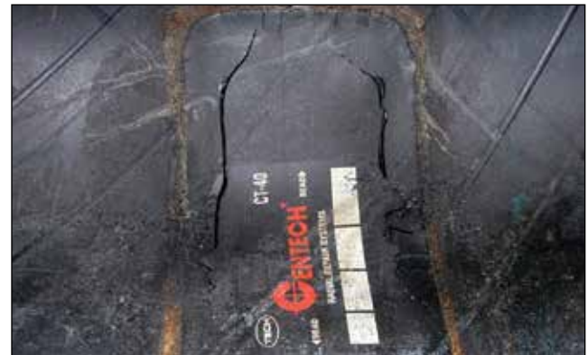
EFFECT: Crack in the Repair Unit CAUSE: Improper Repair or Improper Repair Procedures
